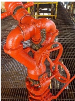
Fire fighting equipment on offshore and land-based drilling rigs.
